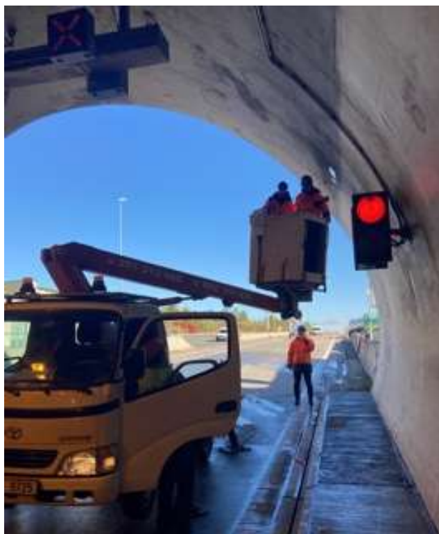
Obr. 8 Instalace BLE zařízení – Cholutice
